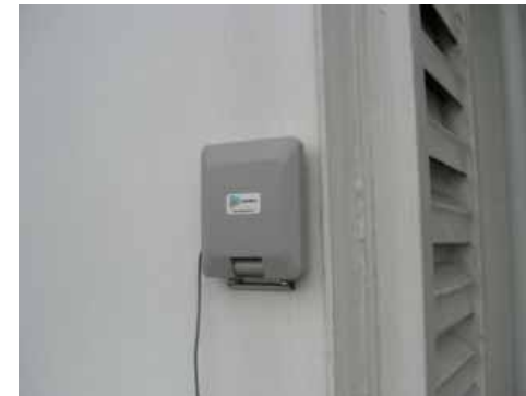
On ship's ventilation duct
